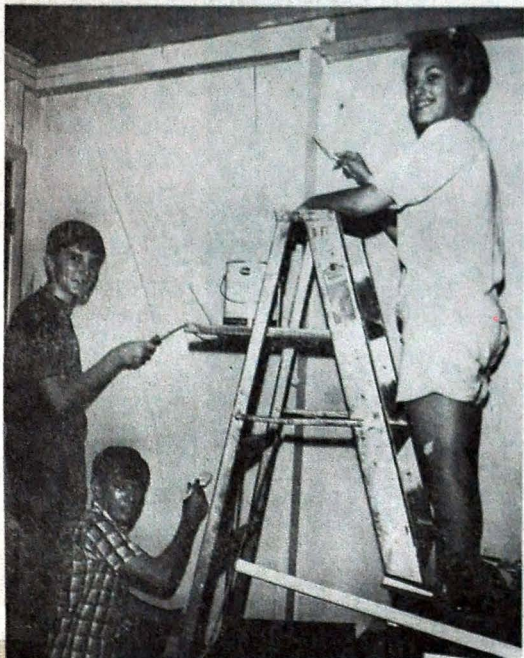
A NEW COAT—Bobby Campbell, Tyner; Steve Harten, Central, and Michele Neshitt of Notre Dame, put on a new coat of paint to the walls of the J.A. Building on Dodds Avenue. Several members are donating their time to renovate the headquarters for this school year.
