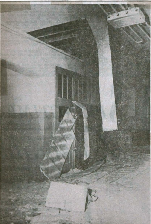
SECTION OF CEILING FALLS AT CENTRAL —Metal laths holding plaster to the ceiling on Central High School's second floor hallway came loose Wednesday and fell to the floor. A portion of the fallen plaster is shown here. No one was injured. The estimated cost of the section will be about $450.—(Staff photo by Delmont Wilson.)
