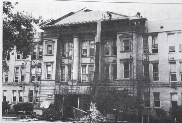
LAST LOOK—This is one of the last pictures taken of Central while her pediment was being removed. Workmen are seen tearing down the brick and wooden super structure.
