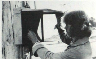
Turn It On — Senior Mike Williams checks fuse box as part of his electrical trade course. Photo by James Gilbert
